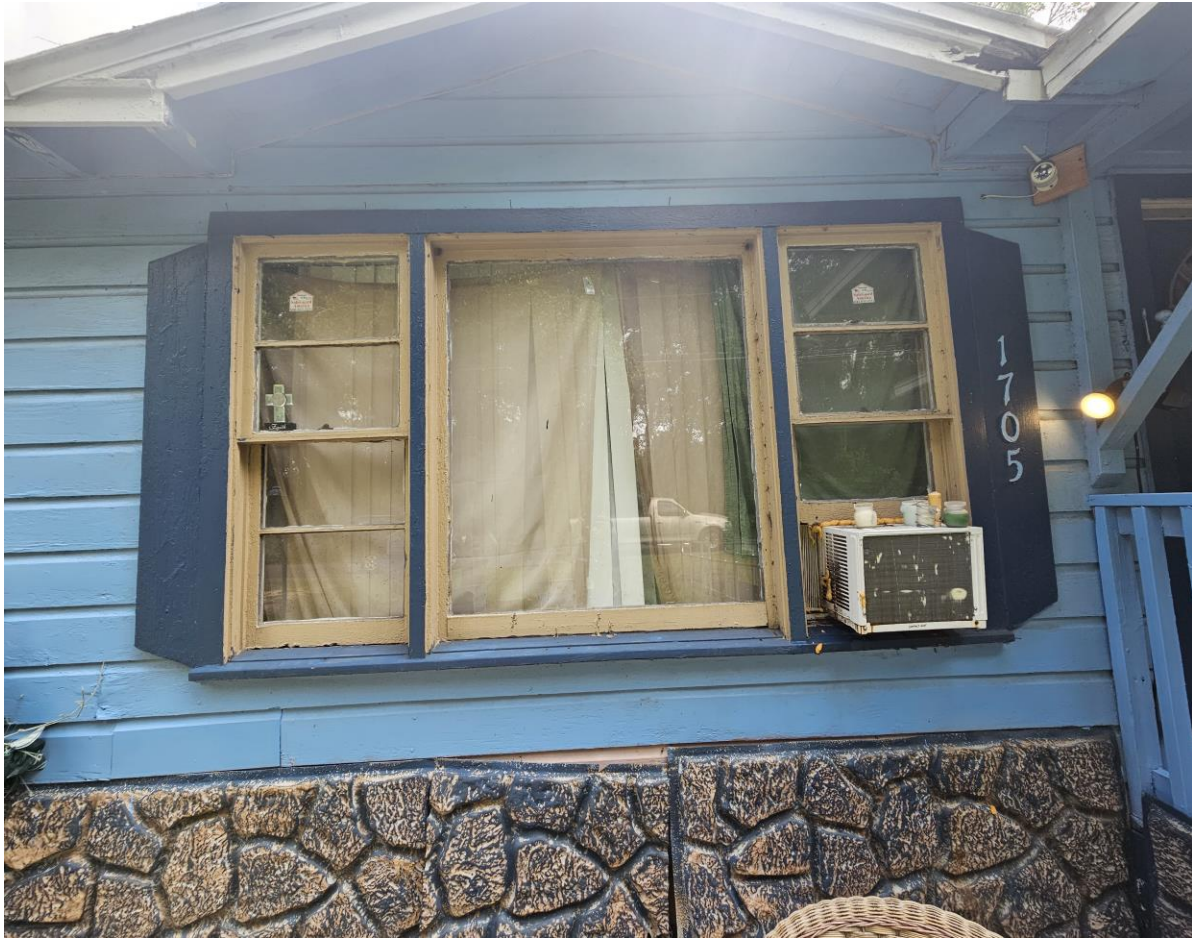
Image 2- View showing example of the existing window and outdated HVAC units.
