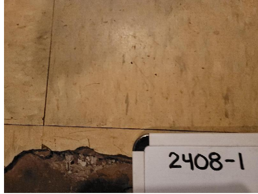
2408-1 12"x12" Floor Tile/Tan (3% Chrysotile) Mastic/Yellow Bedroom A Closet/Pantry (77 sq ft)
