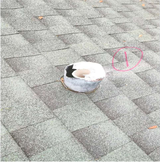
Image 7 - Existing condition - shingle section.
