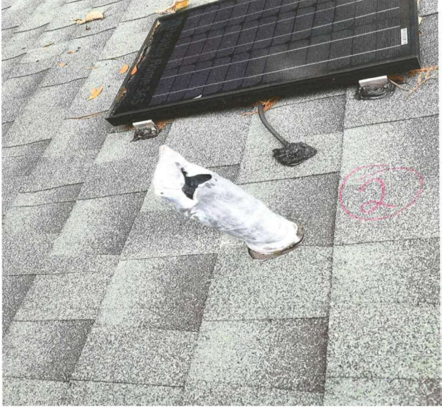
Image 6 - Existing condition - shingle section.
