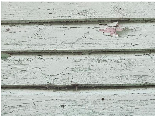
Exterior(008) D-Wall, Center Wood Wall Lead-Positive, Deteriorated
