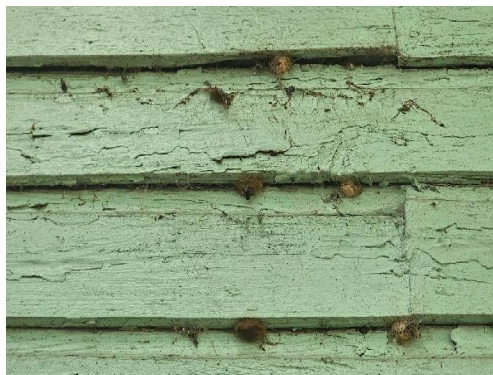
Exterior(008) B-Wall, Right Wood Wall Lead-Positive, Deteriorated
