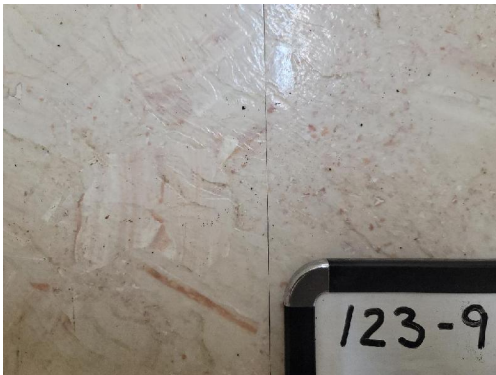
123-9 12"x12" Floor Tile/Adhesive Interior Bathroom Edges
