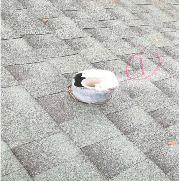
Image 7 - Existing condition - shingle section.
