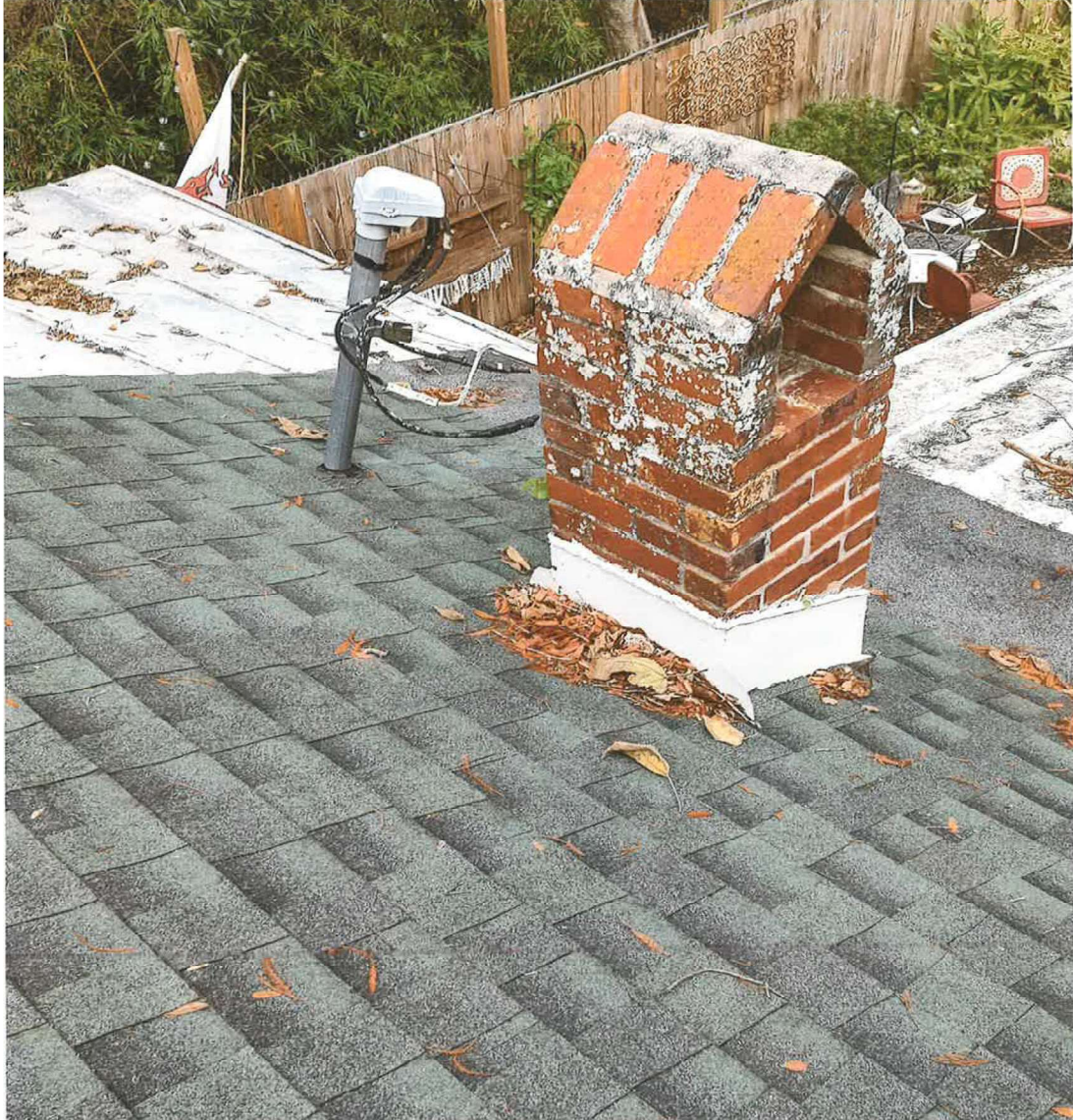
Image 5 - Existing condition - shingle section.
