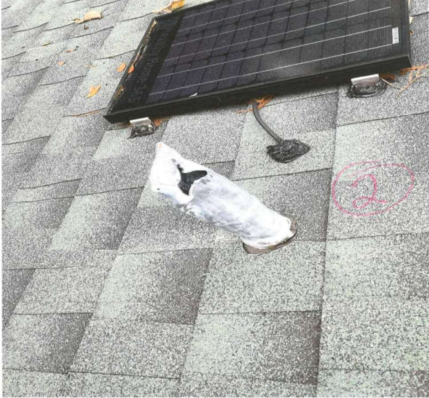
Image 6 - Existing condition - shingle section.
