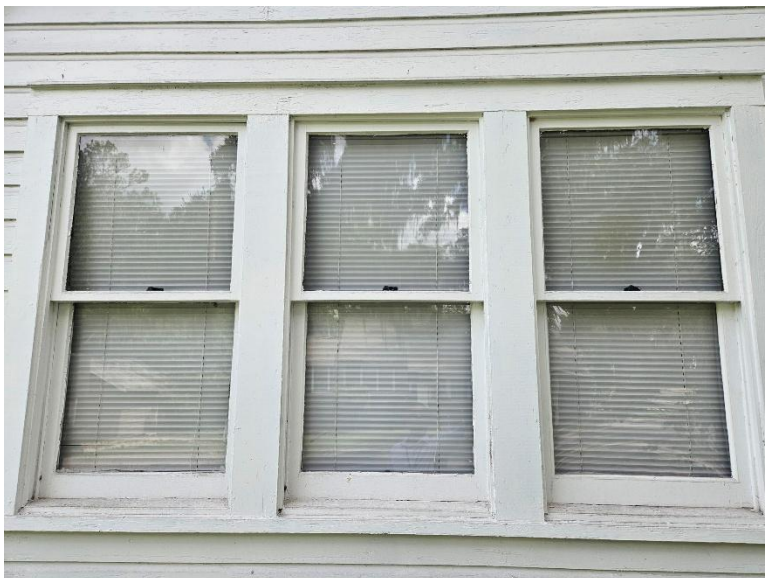
Condition of original windows.
