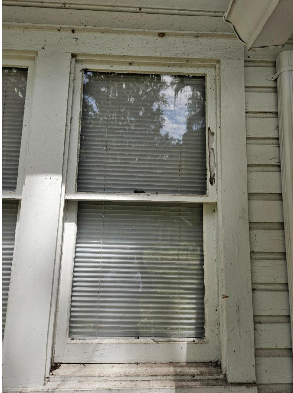
Condition of original windows.
