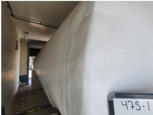
475-1 Tank Wrap/White Typical Interior Tank
