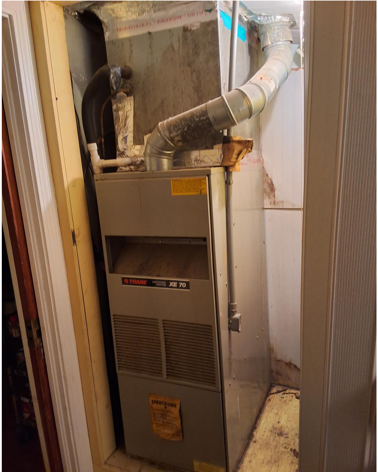
Image 4. Existing HVAC (inside unit)
