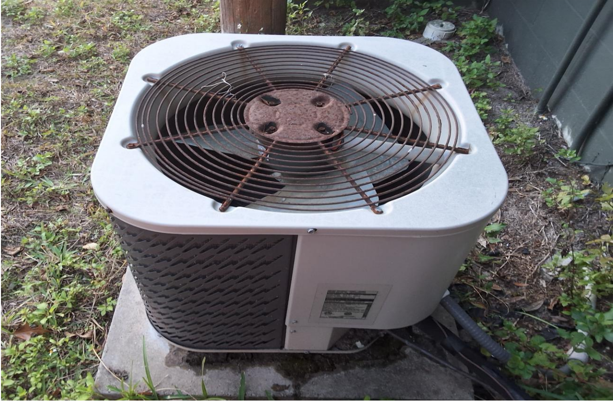
Image 3. Existing HVAC (outside unit)
