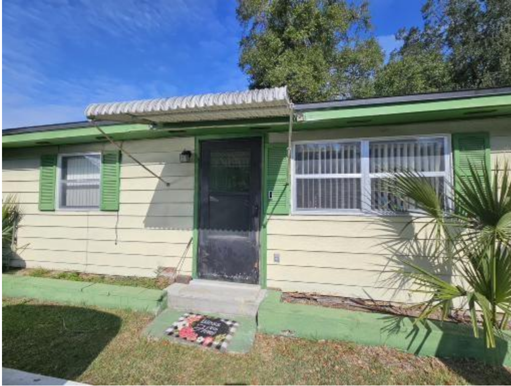
Image 1- Existing conditions of windows at the entrance to the home.
