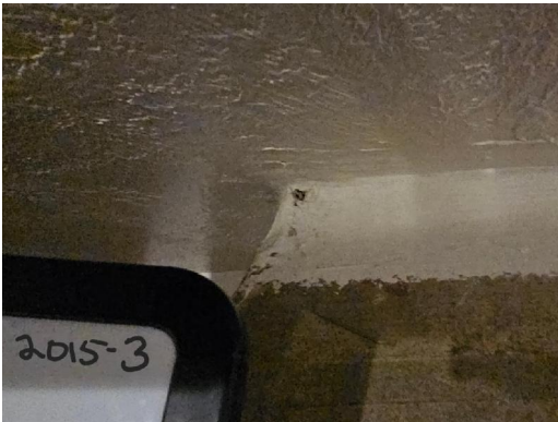
2015-3 Duct Mastic Typical Interior HVAC
