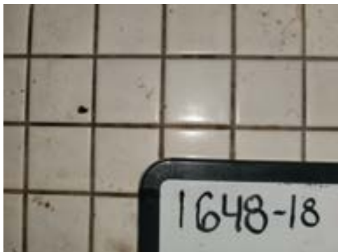
1648-18 Ceramic Tile/Grout Interior Master Bathroom Floor
