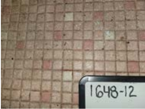
1648-12 Ceramic Tile/Grout Interior Bathroom Floor
