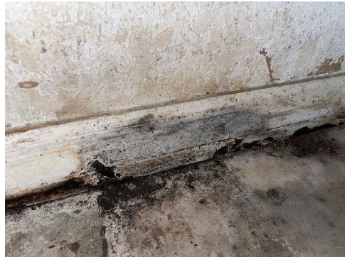
Interior Garage West lower drywall, wood baseboard Visible water damage Visible microbial growth (>10 sq ft)
