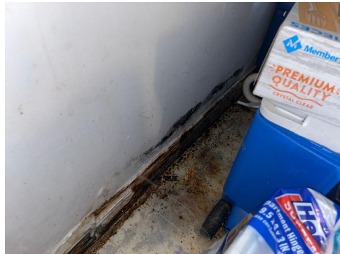
Interior Kitchen South lower drywall, wood baseboard Visible water damage Visible microbial growth (>10 sq ft)
