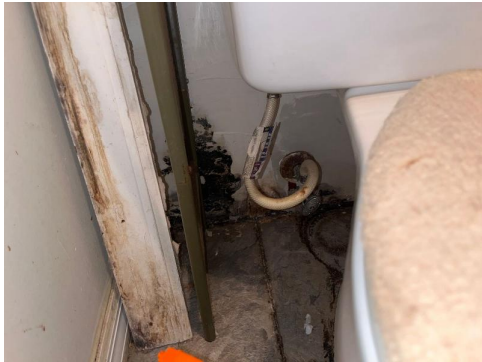
Interior Master Bathroom West lower drywall, wood baseboard Visible water damage Visible microbial growth (>10 sq ft)
