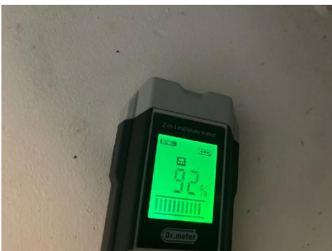
Interior Kitchen South lower drywall wall Elevated moisture content (92%)
