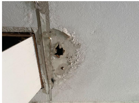
Interior Garage West drywall ceiling Visible water damage Visible microbial growth (>10 sq ft)
