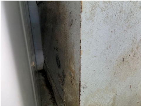
Interior Garage North drywall wall Visible water damage Visible microbial growth (>10 sq ft)
