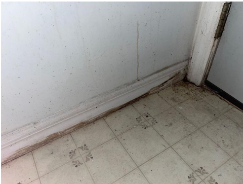
Interior Kitchen East lower drywall, wood baseboard Visible water damage Visible microbial growth (>10 sq ft)
