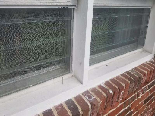
Exterior(012) A-Wall, Left Wood Window Jambs Lead-Positive, Intact
