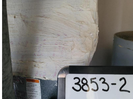
3853-2 Duct Mastic Typical HVAC
