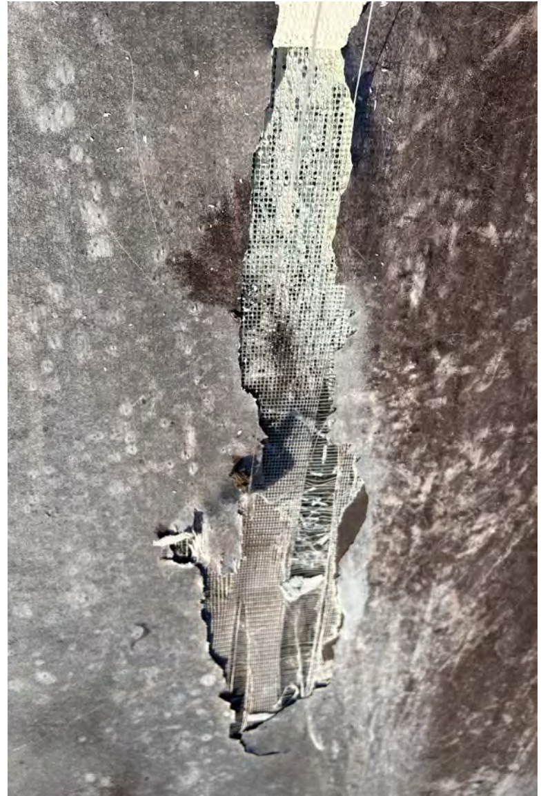
Holes in Membrane
