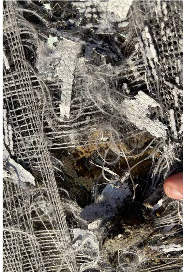
Holes in Membrane
