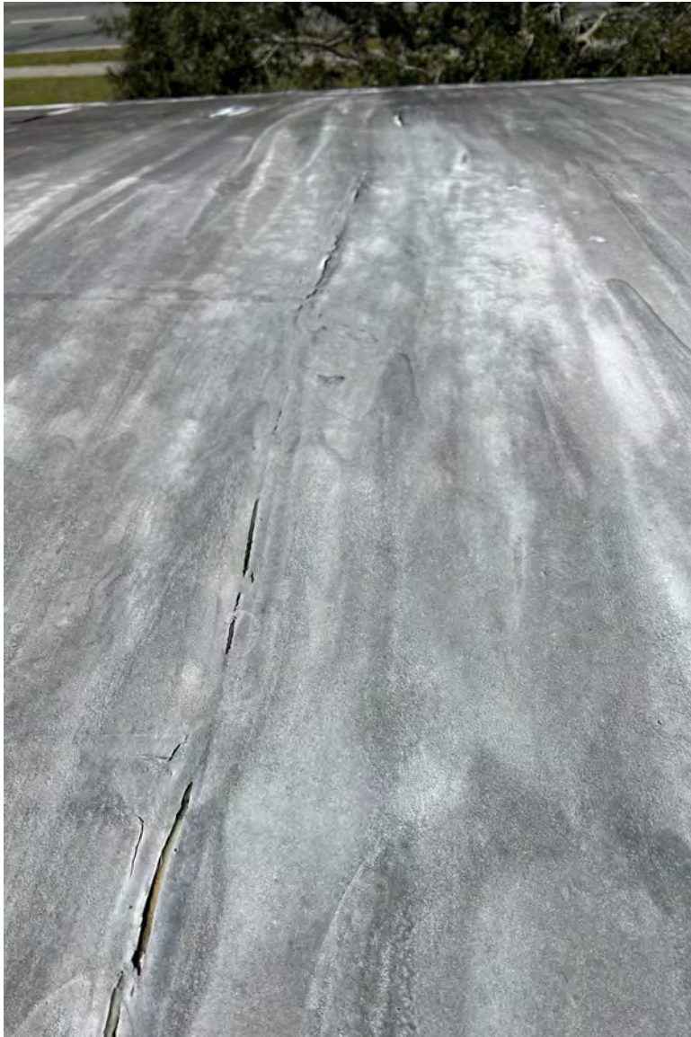
Hole in Membrane
