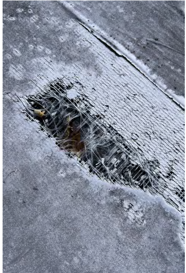
Hole in Membrane
