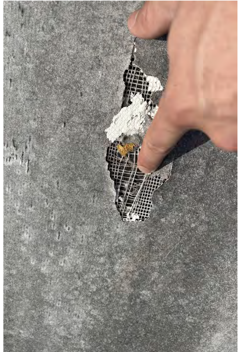
Holes in Membrane
