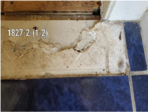
1827-2 Floor Leveler/White/Gray Interior Kitchen/Bathroom
