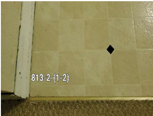
813-2 Rolled Flooring/White Interior Kitchen (80 sq. ft.)
