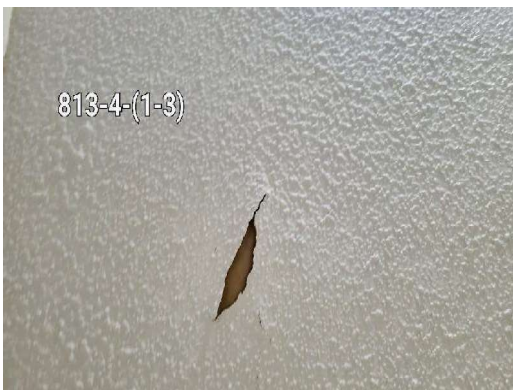
813-4 Ceiling Surfacing Texture/Cream (3% Chrysotile) Typical Interior Ceilings
